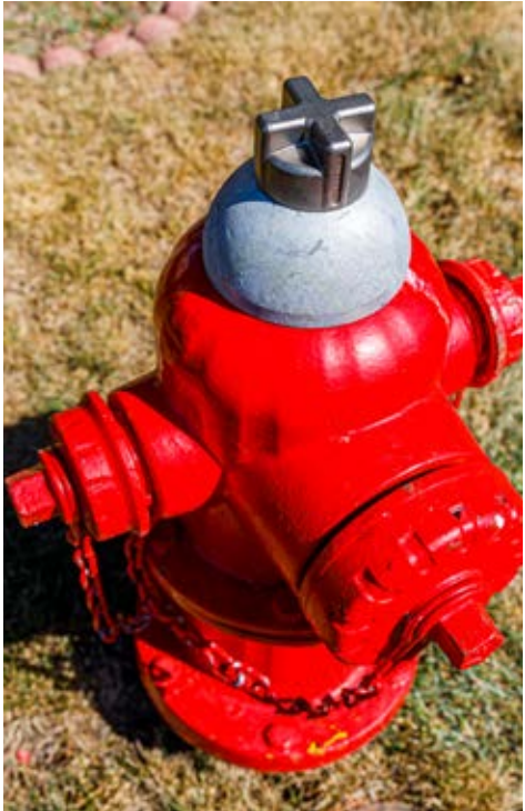
Fire hydrant water lock
