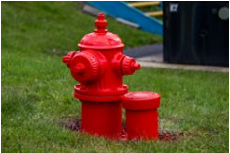
Newly painted fire hydrant
