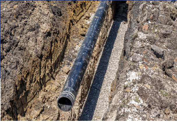
A new section of pipe is carefully lowered into the ditch to be connected to the existing water line and eliminate a dead end.
