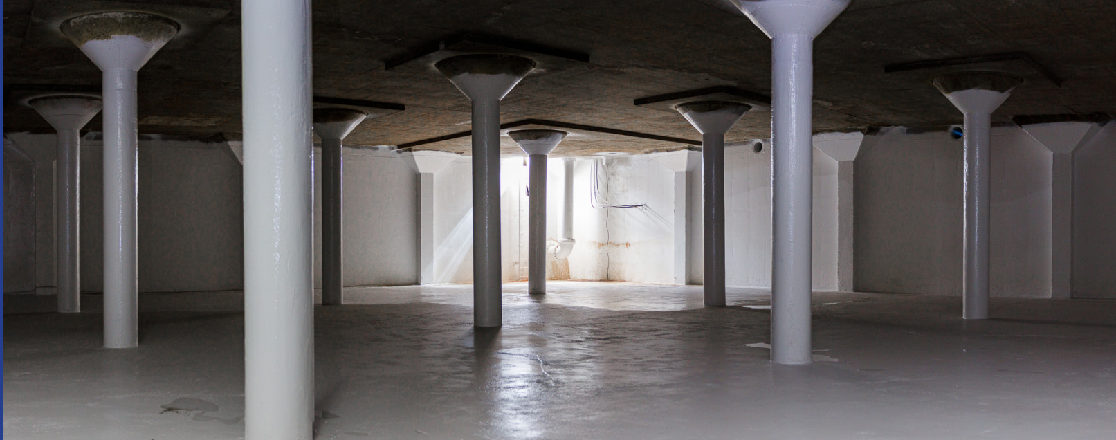
A clean view of the 500,000 gallon underground water storage facility.
