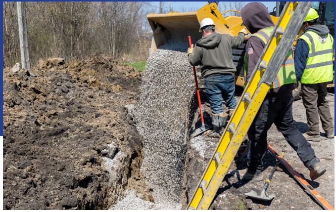
Gravel is poured over the pipe to secure its place in the ground and prepare for the next pipe section to be added.
