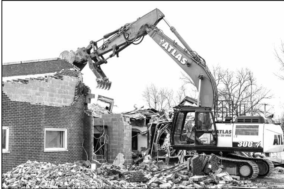
Empty buildings are demolished to make room for the new fueling center.
