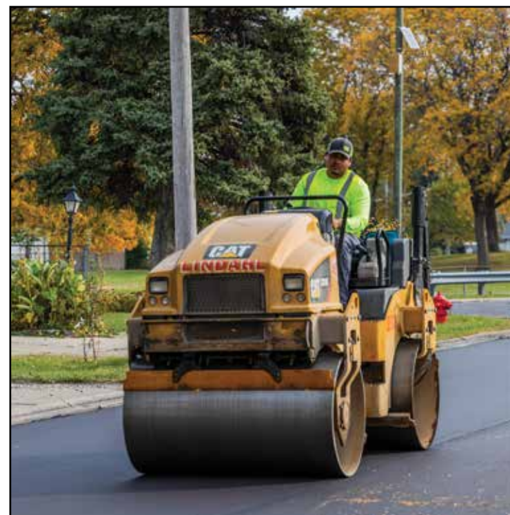
The roller smooths over the remaining asphalt on the cul-de-sac of 81st Place.
