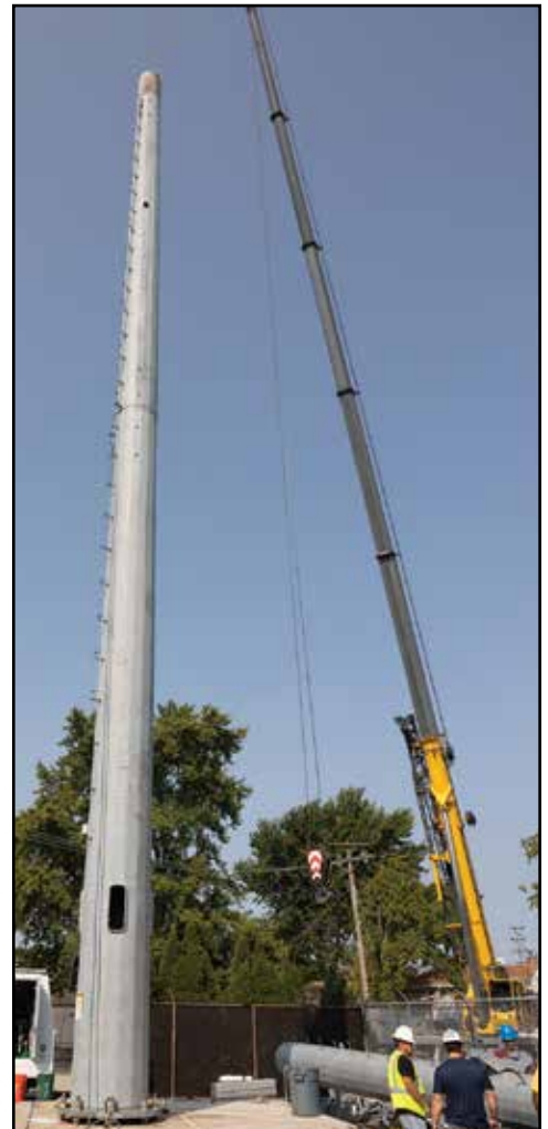
The crane stands ready to lift the cellular infrastructure to the top of the temporary cell tower.
