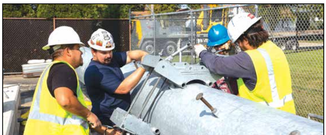
Workers prepare the infrastructure on the temporary tower before it is lifted by a crane.
