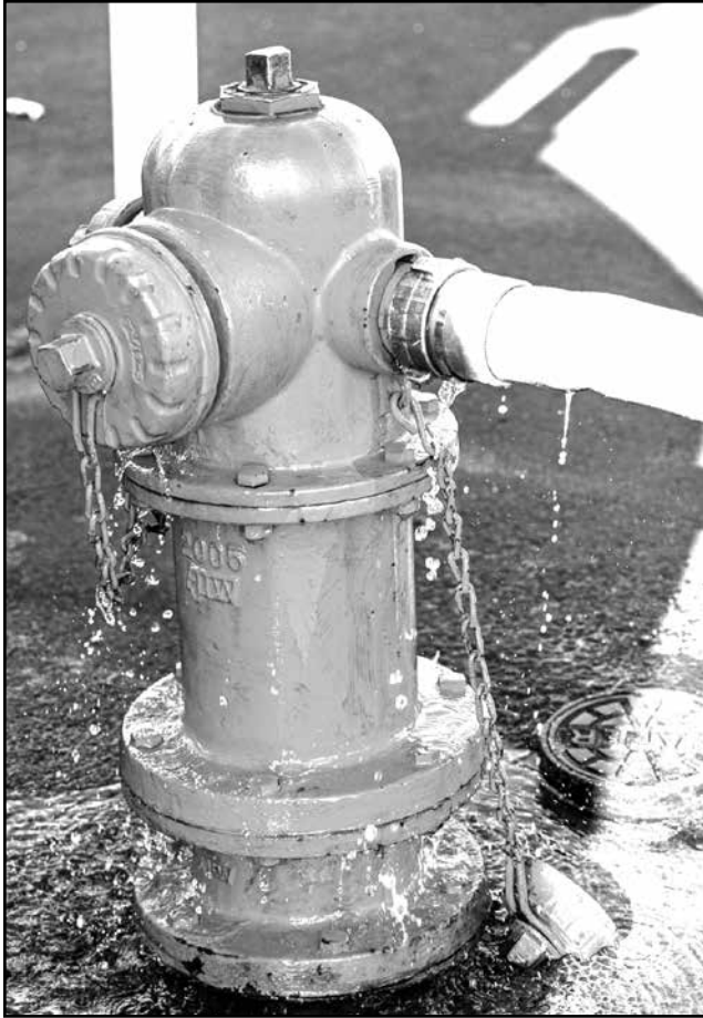
Water flows from a Bridgeview fire hydrant.
