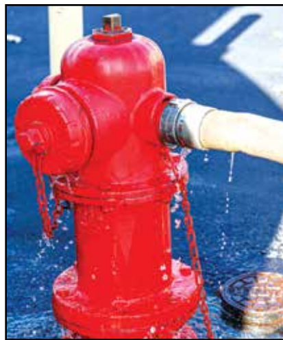
Water flows from a Bridgeview fire hydrant.
