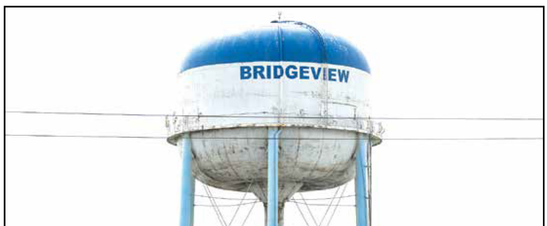
Our water tower will have a new look by the end of 2024.
